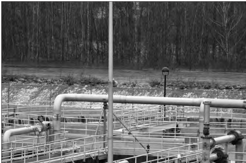
Figure 5 - Pawtuxet River crests the western side of the levee at approximately 1:15 PM on Tuesday, March 30, 2010, and begins flooding the treatment facility. Photo by Peter Ginaitt.
