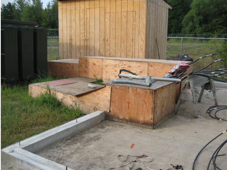
Figure 10: Temporary Switchgear Housing. Photo by Ron Demers.
