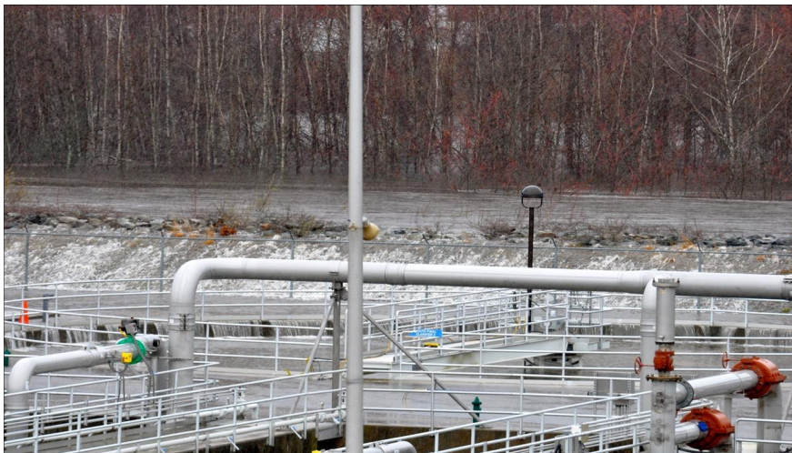
Figure 4: Pawtuxet River crests the western side of the levee at approximately 1:15 PM on Tuesday, March 30, 2010, and begins flooding the treatment facility. Photo by Peter Ginaitt.
