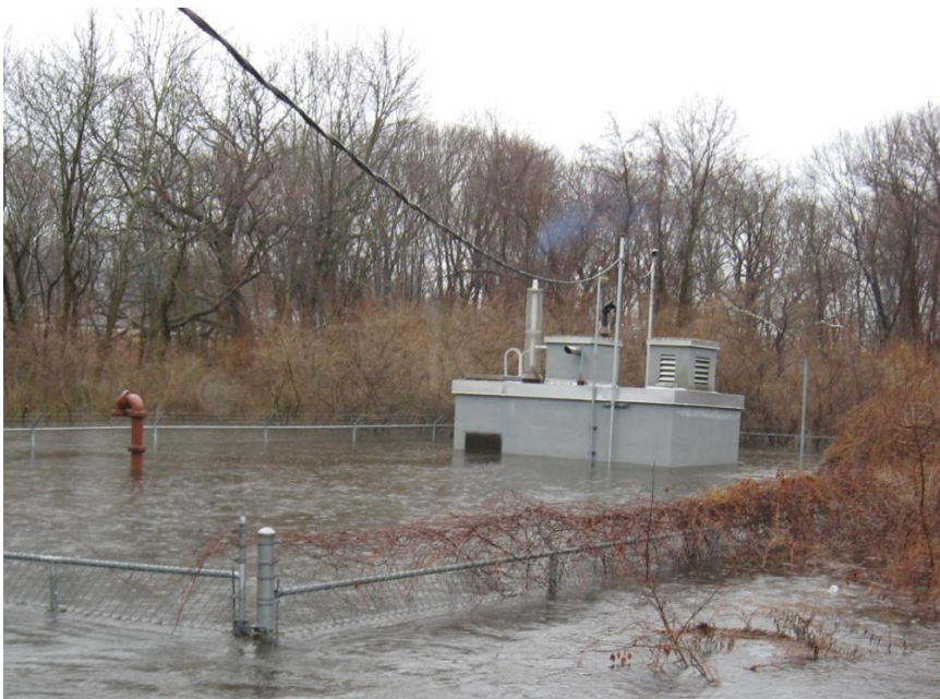
Figure 3: Knight Street Pumping Station, located in a Pawtuxet River floodway, during March 15, 2010 flood. Photo by Patrick Doyle.
